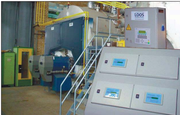
The retrofitted LWA ensures optimum water quality and pays for itself in a very short time
