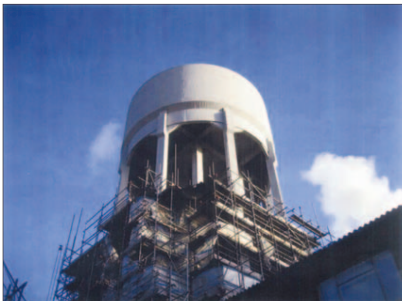
The Sittingbourne water tower was refurbished without disrupting the water supply to the M-real and St Regis mills. The tower supplies process water and water for the fir sprinklers.
